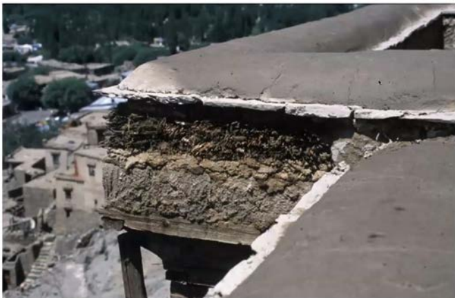
Finished parapet with layers of arga, slate, tamarisk branches, and rammed earth.
